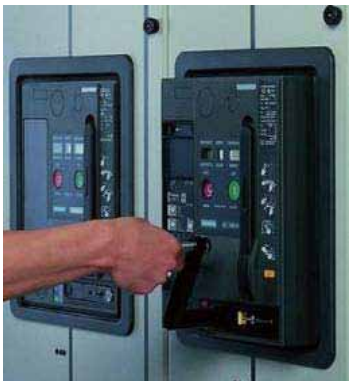
CIRCUIT Breaker DOOR Closed PIX
